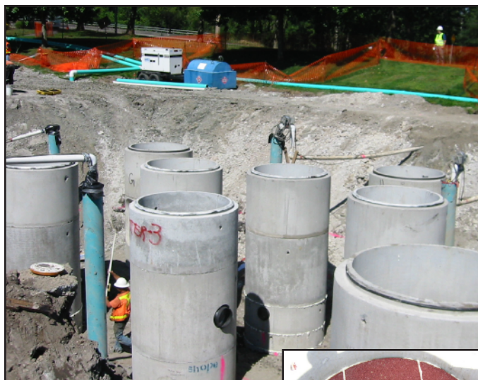
(above) This large water quality treatment train was easily installed in less than one day.
